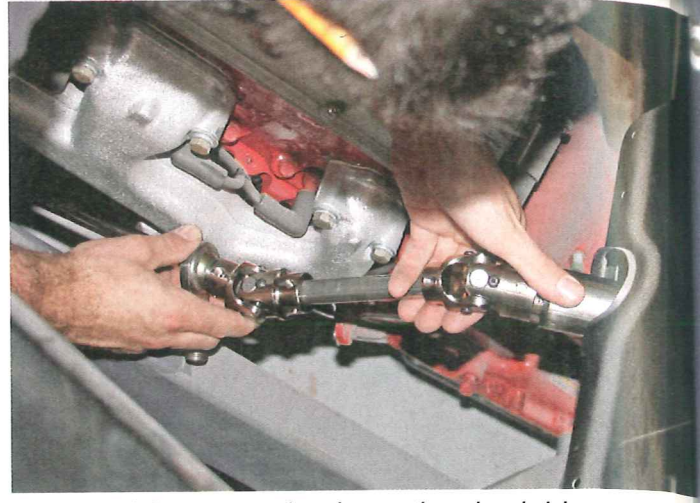
Running the linkage to mate the column to the rack-and-pinion can be tricky for the first timer, but with careful measuring and a little foresight, a three-joint system can be installed in about an hour.
